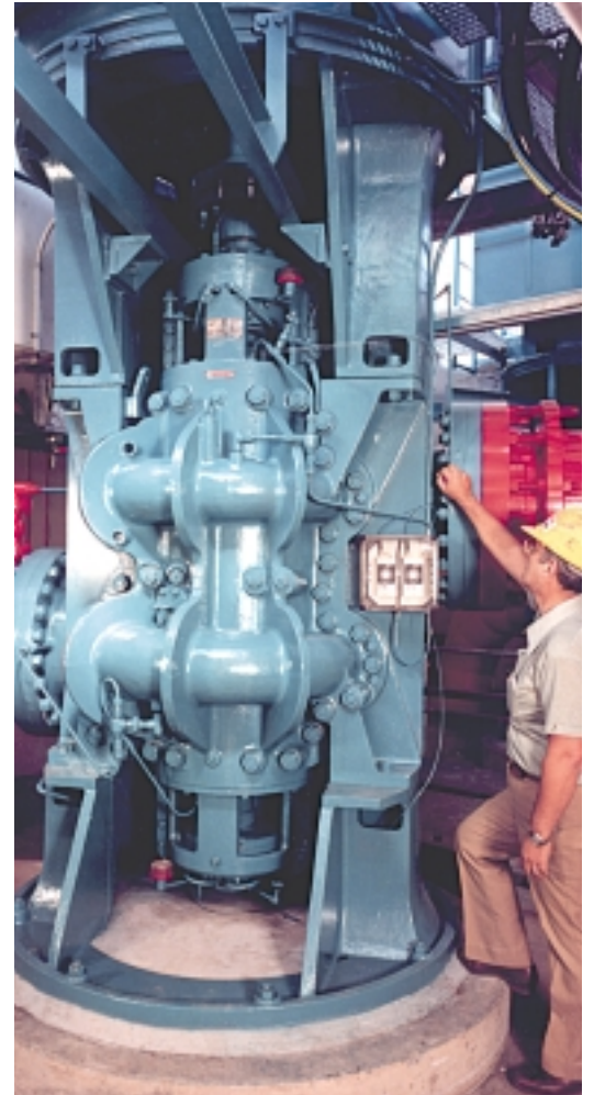
On the right is one of two 600/600 ECS two stage vertical pumps installed for the Toowoomba City Council.
